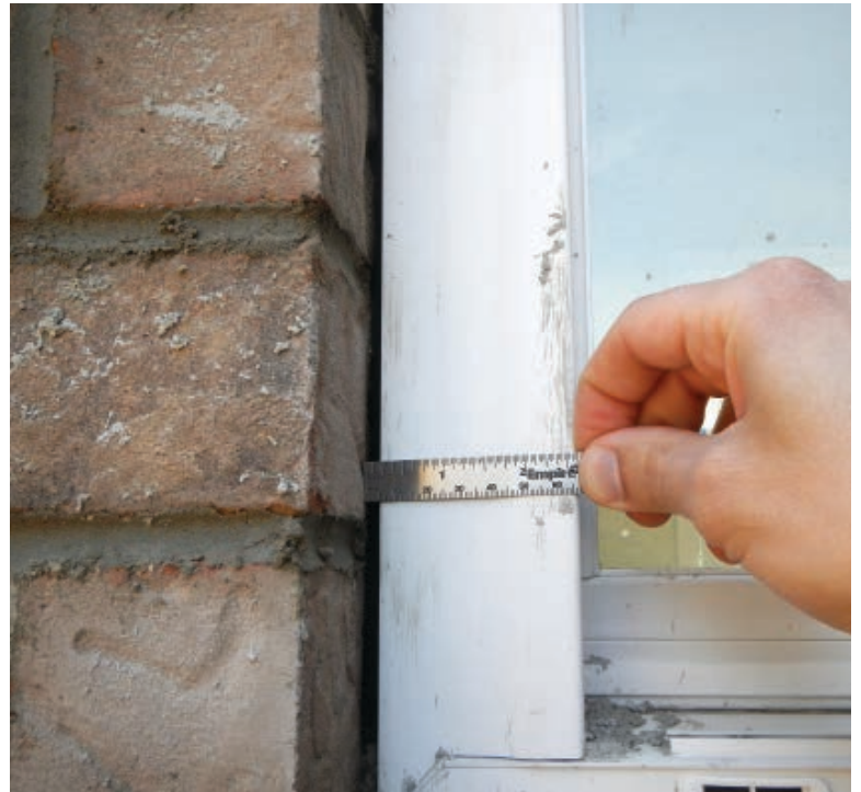
IMAGE 2: BRICK VENEER GAPS
