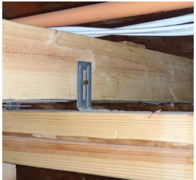
IMAGE 4: TRUSS UPLIFT GAPS
