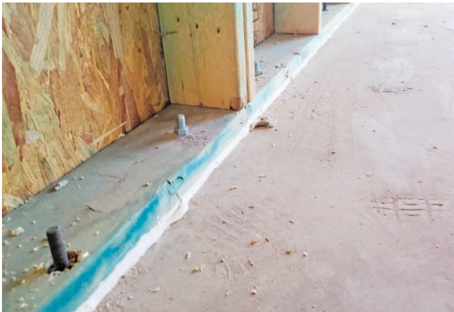
Instead of using expanding spray foam to air-seal sill plates to the subfloor or concrete slab, use a thick, continuous bead of construction adhesive to create a more reliable seal.
