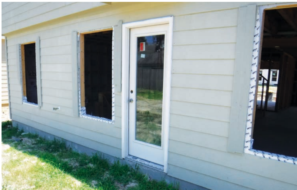
Finish before flashing: To keep working when windows are delayed, it's OK to install the finished siding but hold back the trim so windows can be properly flashed during installation.
