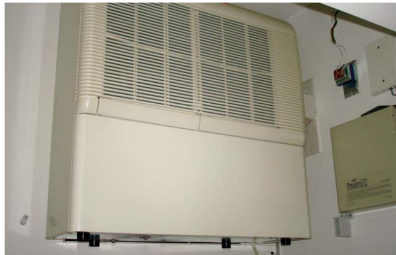
(Above) New dehumidifiers such as this one were installed in all units to avoid future risk.
